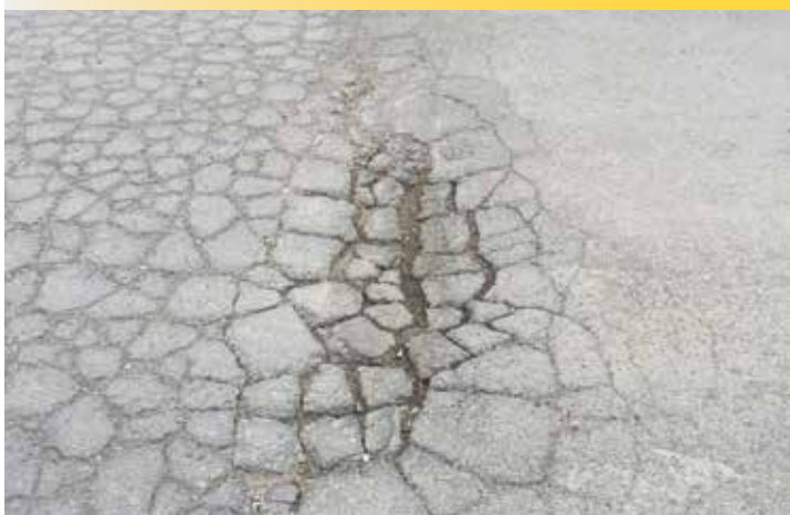
Detects Weight Cracked Areas
