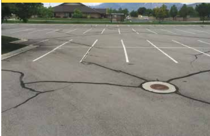
Detects Thermal Cracks
